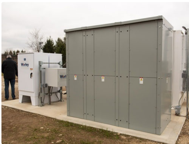
The 137.4 kW solar array and 560 kW/1,200 kWh battery energy storage system will help the Columbus Zoo cut energy costs and reduce its carbon footprint.
