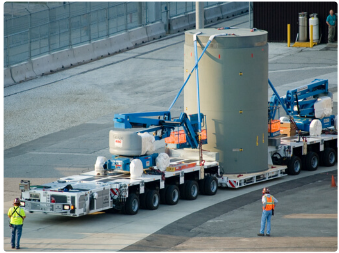
AEP's current spent nuclear fuel cask storage facility can store 94 casks, or 3,008 spent nuclear fuel assemblies.
