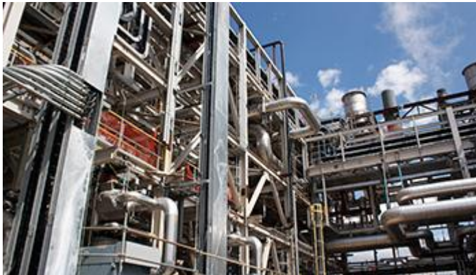
The 580-MW Dresden Plant in Ohio is one of AEP's four combined-cycle gas plants.
