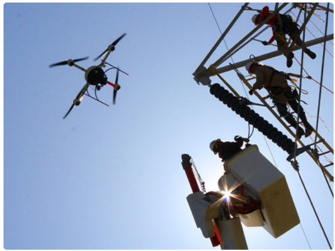
Drones are an effective means of inspecting power lines for regular maintenance and to survey damage after storms.
