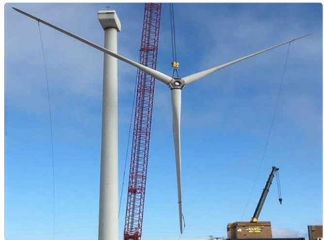
In 2018, AEP Renewables formed a joint partnership to re-power roughly 350 MW at two previously wholly-owned Texas wind farms, Desert Sky and Trent Mesa.
