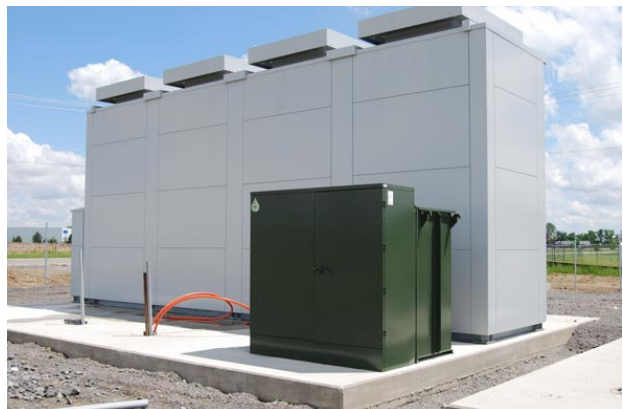
AEP's Electric Transmission Texas' 4-MW NAS ® sodium sulfur battery system located in Presidio, Texas.
