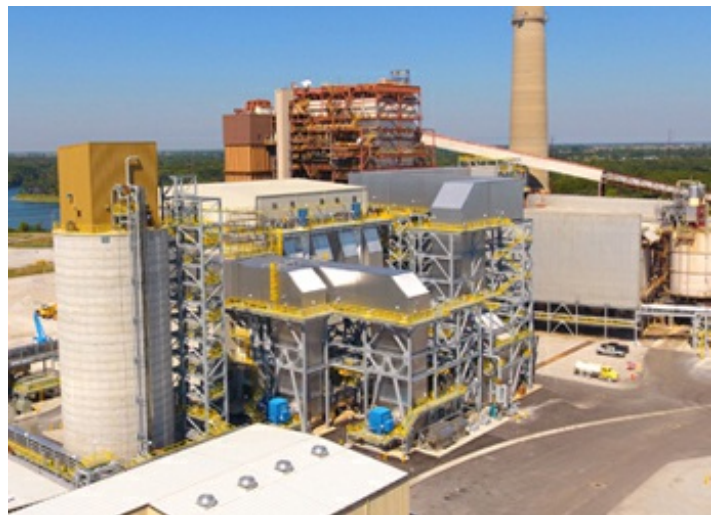
New environmental equipment at Flint Creek includes (left to right) the lime silo, NID/baghouse scrubber unit, exhaust duct to stack (above existing precipitator) and by-product silo.
