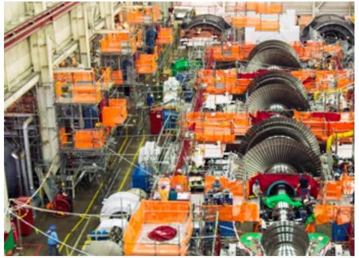
The Cook Nuclear Plant's Unit 2 turbine replacement project was the plant's biggest Life Cycle Management project; its new three low-pressure and high-pressure turbine rotors will increase generation output at certain times of the year.
