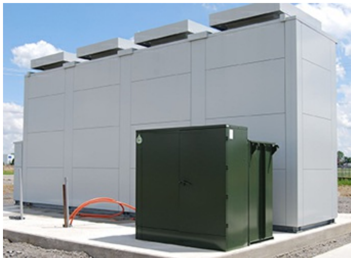
Energy storage can sometimes be the most cost-effective, efficient solution to a reliability issue.
