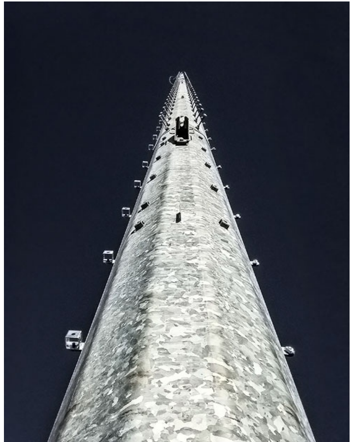
Looking up at the 120-foot pole at Elcona Station in Elkhart, Ind. The station is part of Indiana Michigan Power's volt var optimization project, a distribution automation system.
