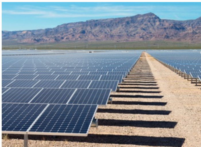
Boulder Solar II is a 50-MW-AC solar facility in Nevada that began commercial operation in January 2017.
