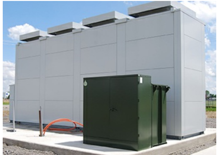
Energy storage can sometimes be the most cost-effective, efficient solution to a reliability issue.
