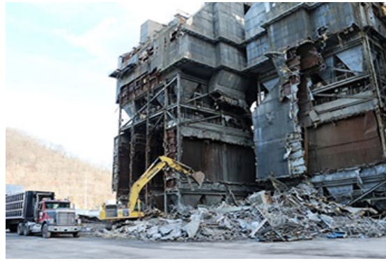
Appalachian Power’s Clinch River Plant began removal of the three precipitators at the plant that were installed in 1975 to remove more than 99 percent of dry ash from the exhaust gas produced by the Plant’s coal burners. Two of the plant’s three coal units have been converted to natural gas; one unit was retired in 2015.
